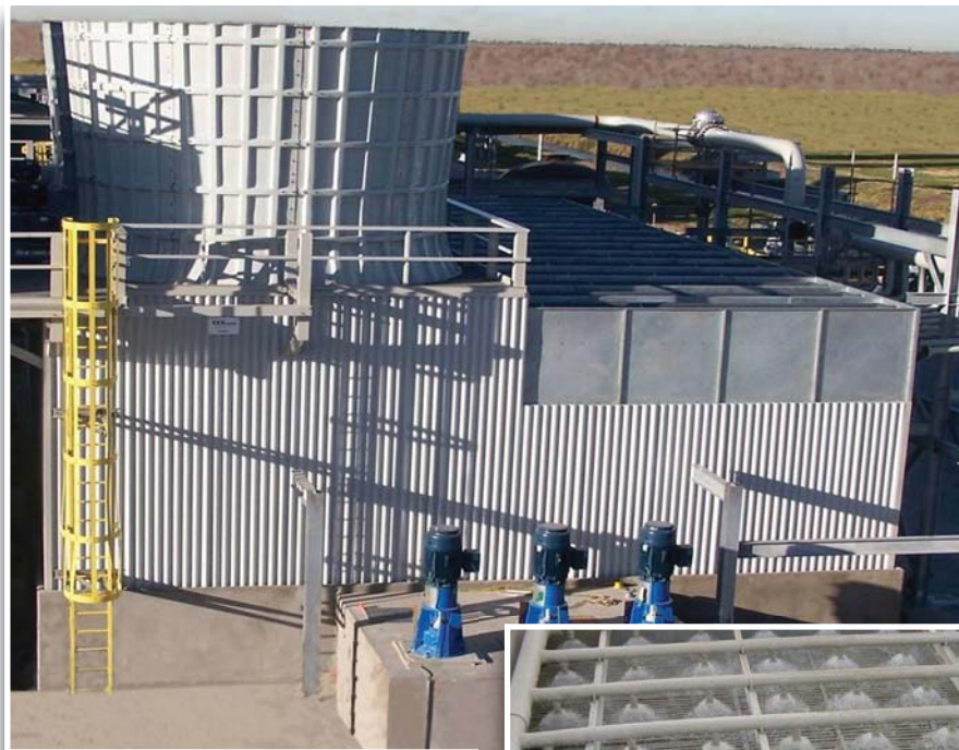
Field erected Wet Surface Air Cooler.
