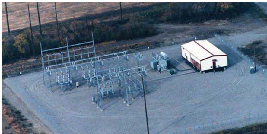
Severe climate installation.
